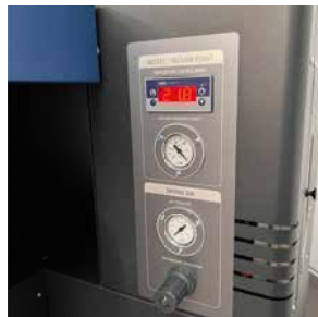
Drying- and vacuum controls
